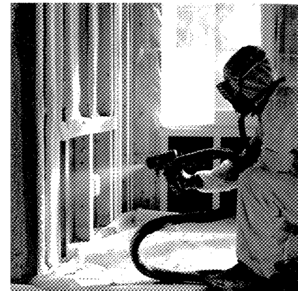
Proper prep yields the best installation. While spray foam installed by a pro, it's your responsibility to prep the site. Mask windows, electrical boxes, and even floors is important if you want the foam contained to wall, roof, and floor cavities. Anyone during the installation should be outfitted for optimum protection.
